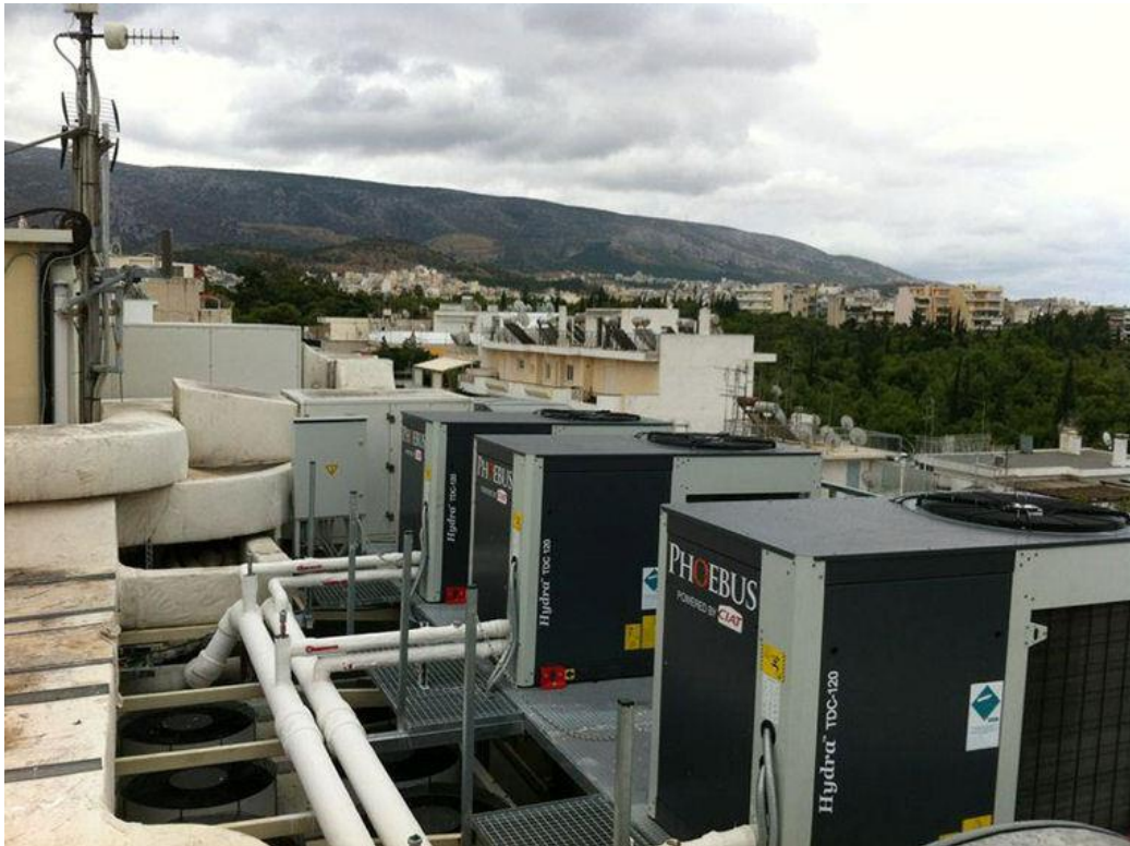
Figure 10 – Hydra @ Crowne Plaza Athens, Greece
